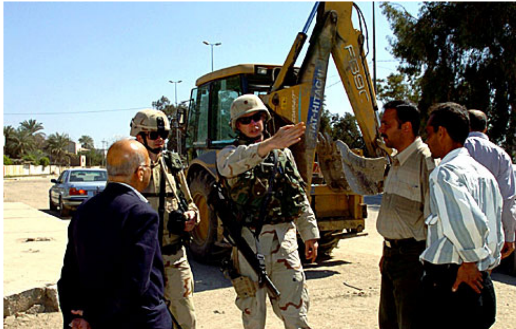
Much of the reconstruction work in Iraq is being carried out by local contractors, here under the supervision of personnel from the U.S. Army Corps of Engineers. PHOTO: CPO EDWARD MARTENS/U.S. ARMY CORPS OF ENGINEERS
