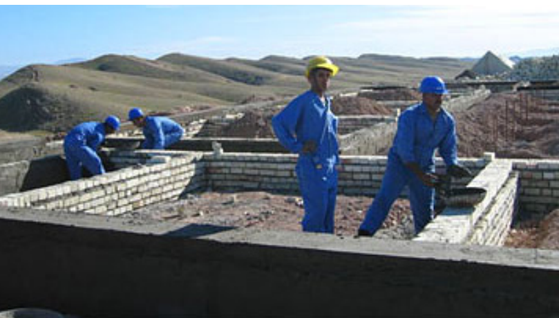
Important construction work on border forts is being conducted by local Iraqi contractors.
